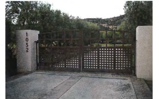
Vehicular Swing Gate 5
